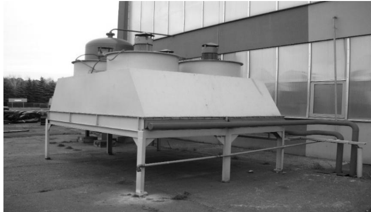
Fig. 7.8. Heating oil cooler of vulcanizing presses - present state
