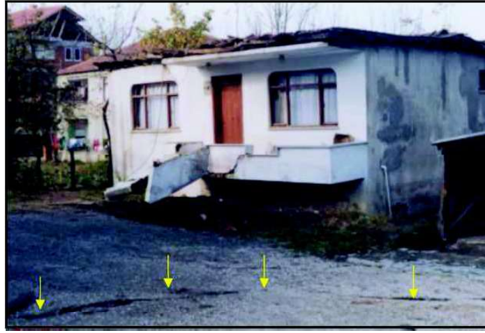
Fig. 16. The view of embedded the building with one storey after the liquefaction induced Duzce earthquake 1999 [Demirtaş et al, 2000]
