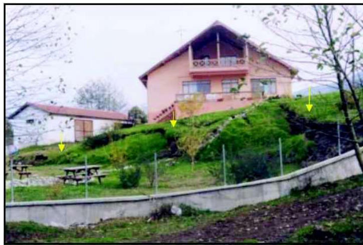
Fig. 15. Ground movement displacement of 1.4 m right side sliding between wall of garden and pool channel in Golormani [Demirtaş et al, 2000]
