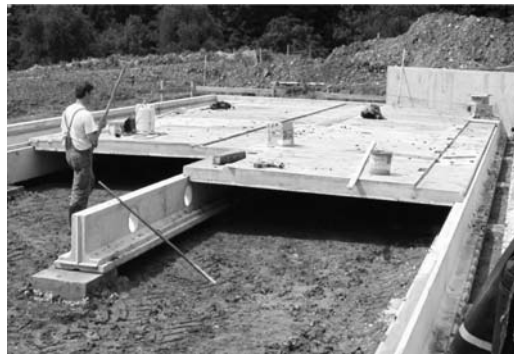
Figure 1: Prefabricated floor plate forming together with the lateral slurry channels, the central wall and the soil a cavity
