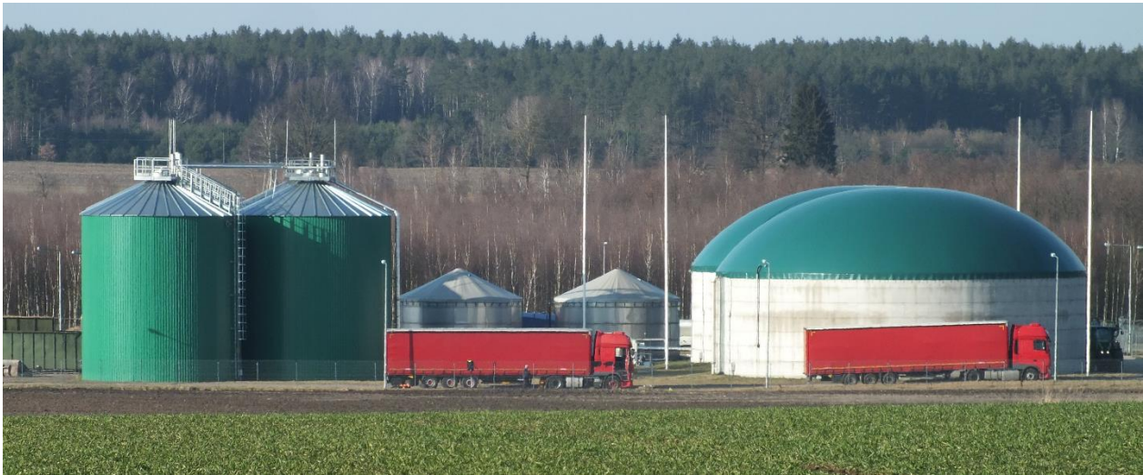
Fig. 1. Agricultural biogas plant (Dynamic Biogas technology) in Jaromierz
