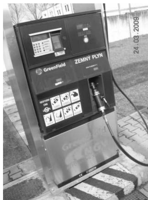
Fig. 1. CNG dispensers - Greenfield A.G.
