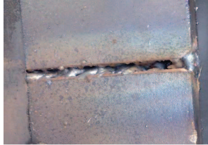
Fig. 7.2. Incomplete filling of the weld groove.
