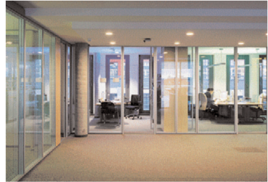
The primary aim of this project was to produce 'good individualized office lighting.' The idea of the RGB luminaire was to replicate the dynamic quality of daylight through the variable composition of luminous colours and light intensities with a high-tech luminaire design. The pictures depict different "lighting moods" produced by indirect lighting components.
