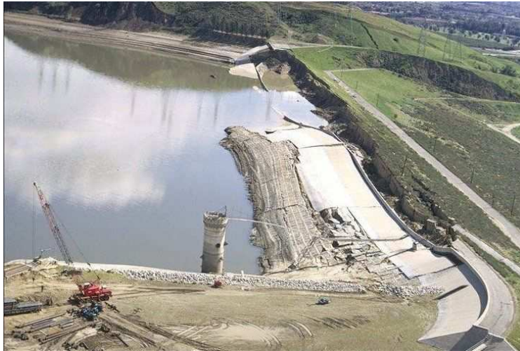
Fig. 19. Dam failure due to embankment liquefaction after seismic event – San Fernando, California, February 1971
