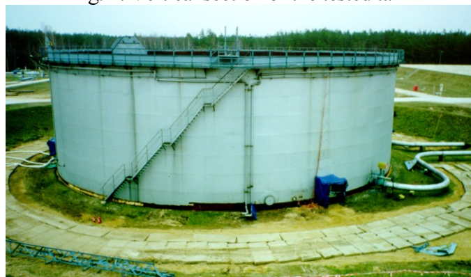
Fig. 2. General view of the tank
