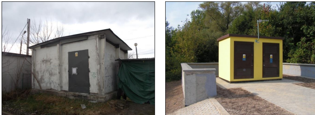
Fig. 1. Examples of transformer stations in the area of Krakow (Source: own materials)
