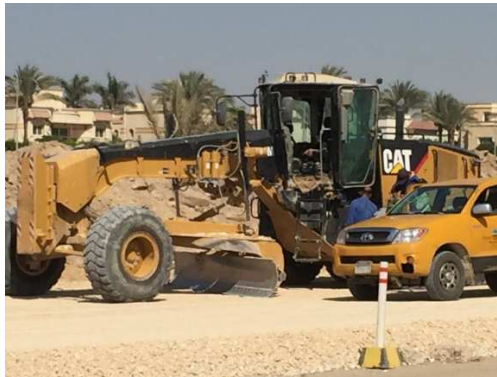
Fig. 10. Waiting for mechanical problems
