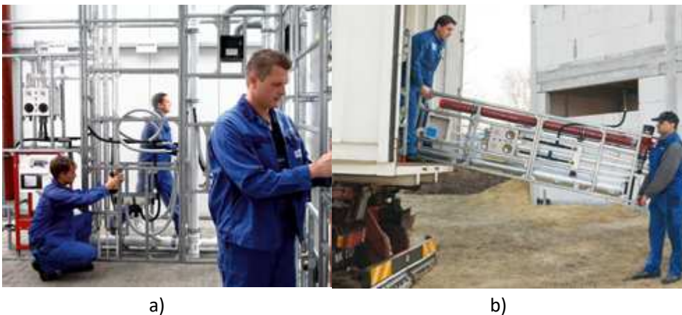
Fig. 2. Prefabricated TECE wall modules a) extended system of wall modules, b) transport to the construction site
