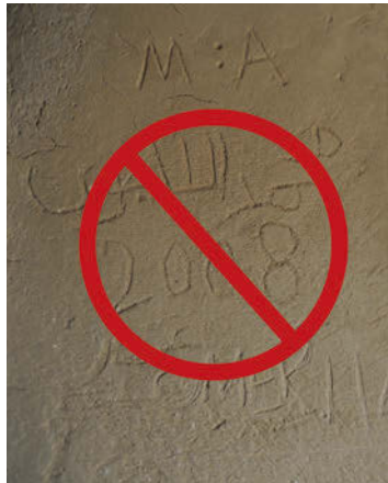
Writing on the walls permanently hurts the heritage of Old Dongola (Photo T. Fushiya)
